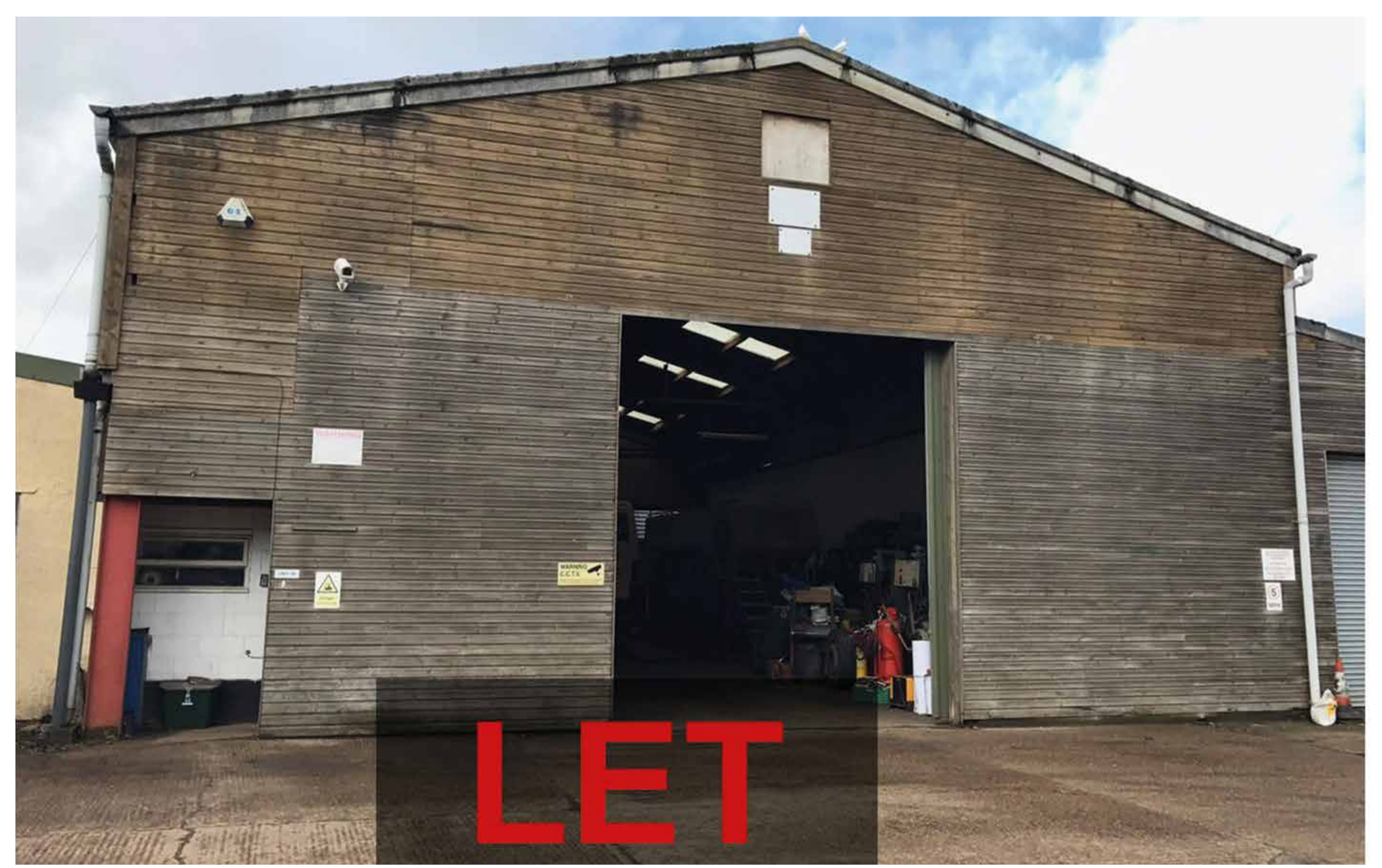
MUCH OF WEALDEN'S LOGISTICS SPACE IS IN POOR QUALITY CONVERTED FARM BUILDINGS
